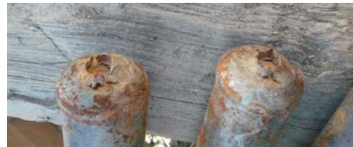
Failure of spikes on poles due to poor quality welding and not passing into pole body.
