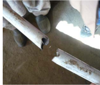
Pole failure under snow load. This pole was weakened as a result of the hole for vertical support, Allai valley.
