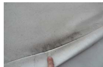
Detail of seam showing where stitching was causing water to collect.
